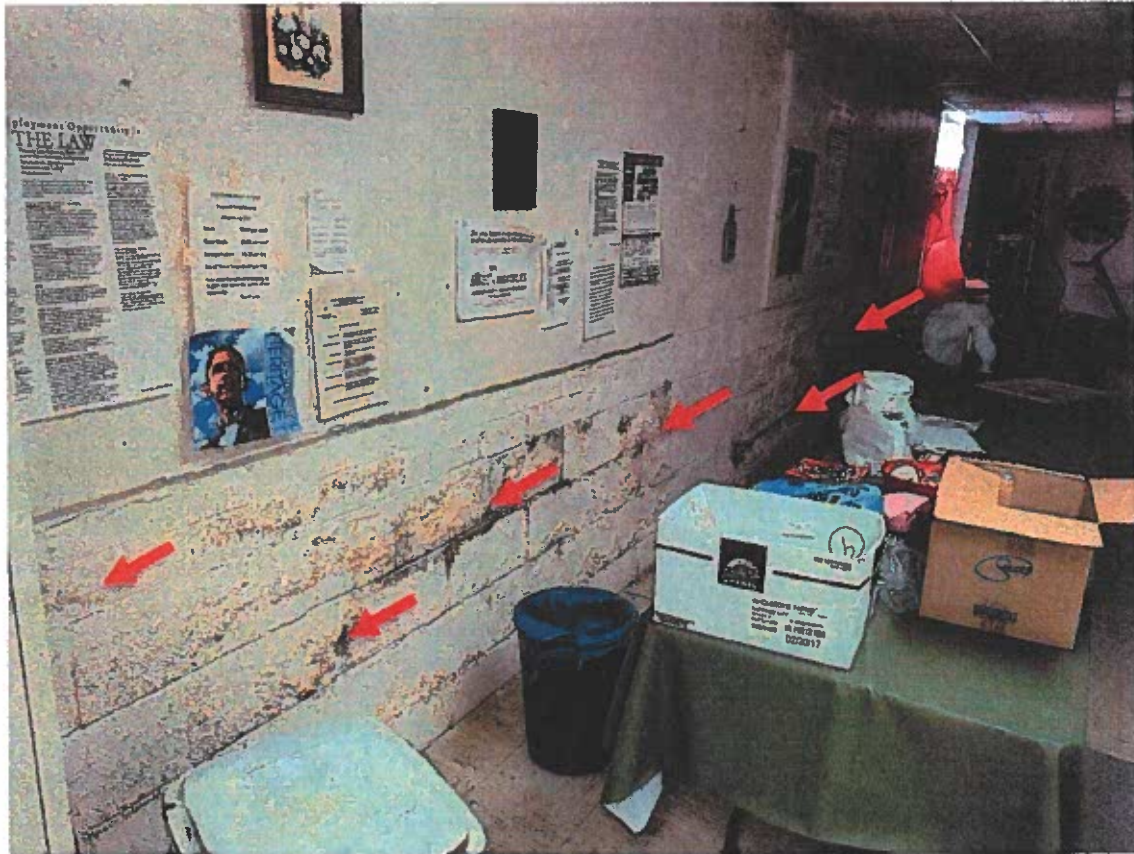
Figure 2: Interior side of an exterior wall. Moisture stains and efflorescent salts (red arrows) were observed at several locations within the building due to roof damage and/or improper or damaged waterproofing at the roof perimeter and framed window openings.
