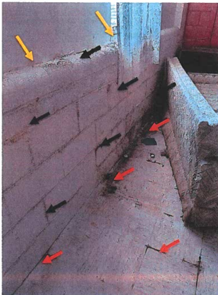
Figure 4: Interior side of an exterior wall. Moisture stains and efflorescent salts (black arrows) were observed at several locations within the building due to roof damage and/or improper or damaged waterproofing at the roof perimeter and framed window openings. Flooring damage (red arrows) at the base of walls was observed adjacent to many of the exterior CMU walls. Window sill and gypsum wallboard moisture damage (yellow arrows).
