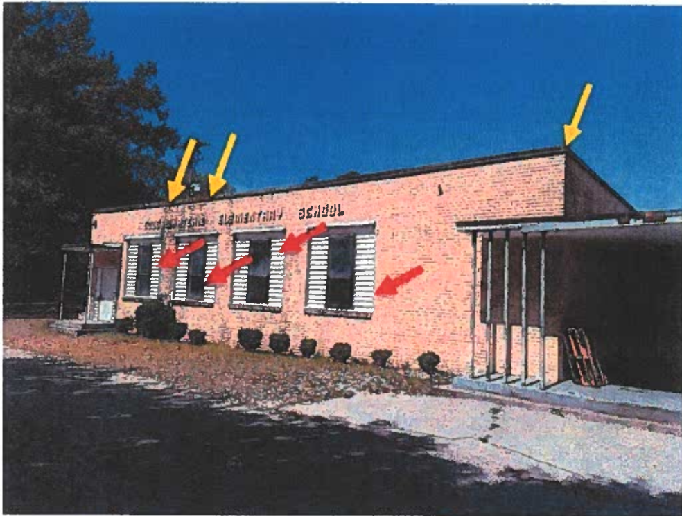
Figure 1: Typical exterior wall elevation. Yellow arrow showing flashing and long-term roof damage. Moisture is most likely entering into the CMU wall/roof flashing along the roof perimeter. Red arrows at stud-framed window openings and windows where moisture is entering the building. This appeared to be a systemic issue due to the lack of proper waterproofing at these locations. The roof and flashing will need isolated repairs or the roofing system replaced. The windows and framed window openings will need to be removed and designed by a registered architect. The newly designed framing and waterproofing will likely require new windows meeting the latest code requirements.
